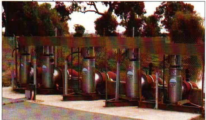
Four model 14/16's and one model 11/14 with a total output of 1760 litres/second, and 5 metres Total Dynamic Head as part of an automatic drainage control system for local government.
