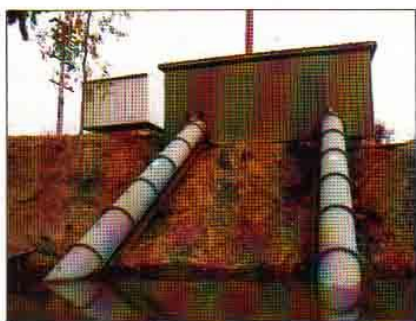
An exterior view of the river pump station on the Murrumbidgee River, NSW, Australia.
