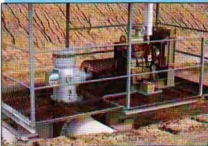
The model 21/24 recirculation system pumping 900 litres/second with 6 metres Total Dynamic Head with below ground discharge at Moree, NSW Australia.
