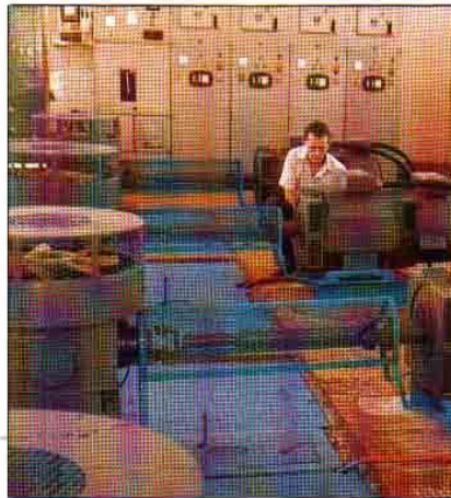
3 model 11/14 pumps operating at Alor Star, Malaysia.
