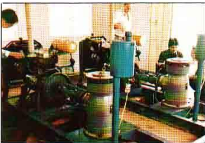
Three model 11/14s commissioned for the Department of Irrigation and Drainage, Perak, Malaysia.
