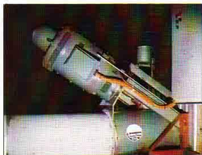
The model 21/24 Angle Application Pump with hollow shaft and electric motor drive, operating at Akuna farms, Darlington Point, NSW, Australia. Pumping 1200 litres/sec with 8 metres Total Dynamic Head.
